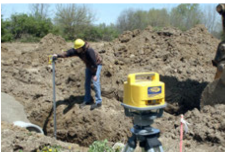
Eliminate dangerous over the trench and in trench grade checks
